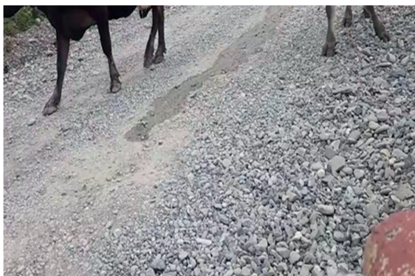
Figure 3. An example of a poorly finished track, note the variety of stone size and lack of compaction on the top layer.
