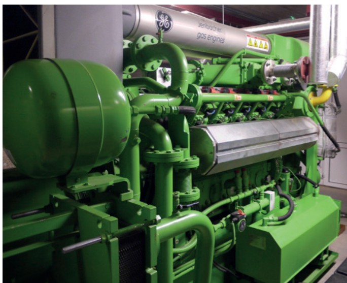
Figure 7: Combined heat and power (CHP) engine
