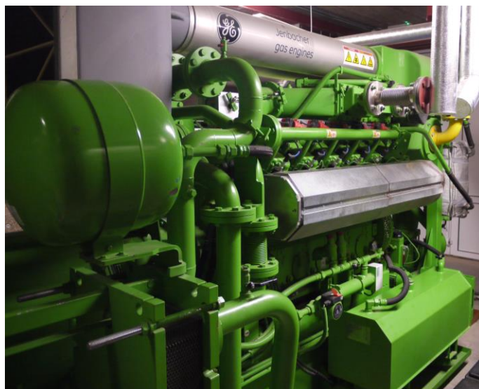
Figure 7: Combined heat and power (CHP) engine
