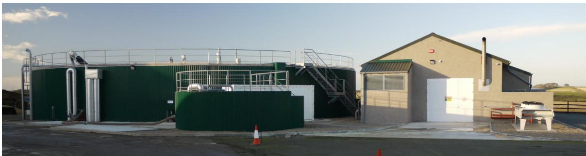
Figure 1: Farm AD installation
