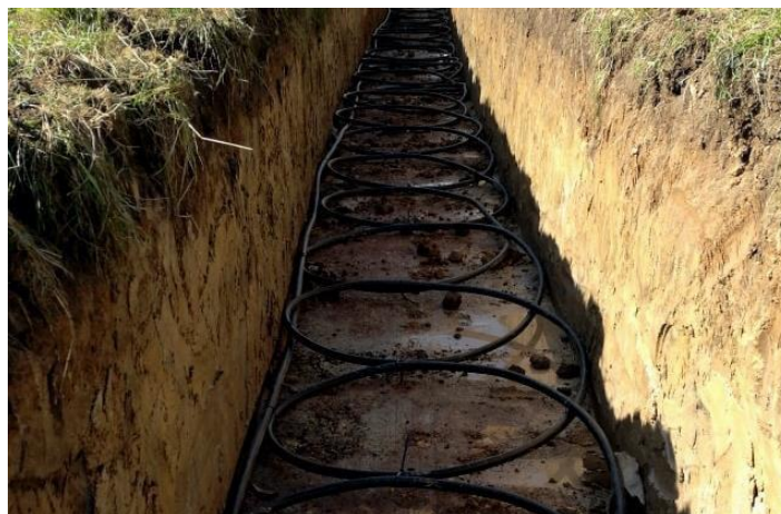
Figure 4; horizontal ground collector with “slinkies”
